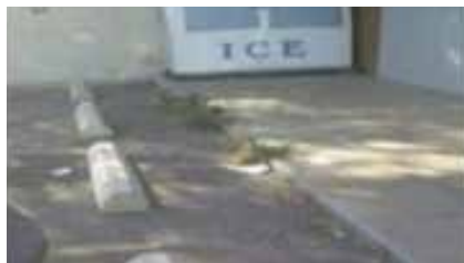
Weeds visible from more than 5' away
