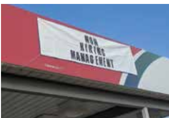
Unapproved signage on canopy
