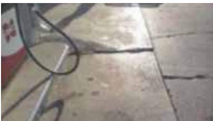
More than two cracks 1" deep and 12" in length
